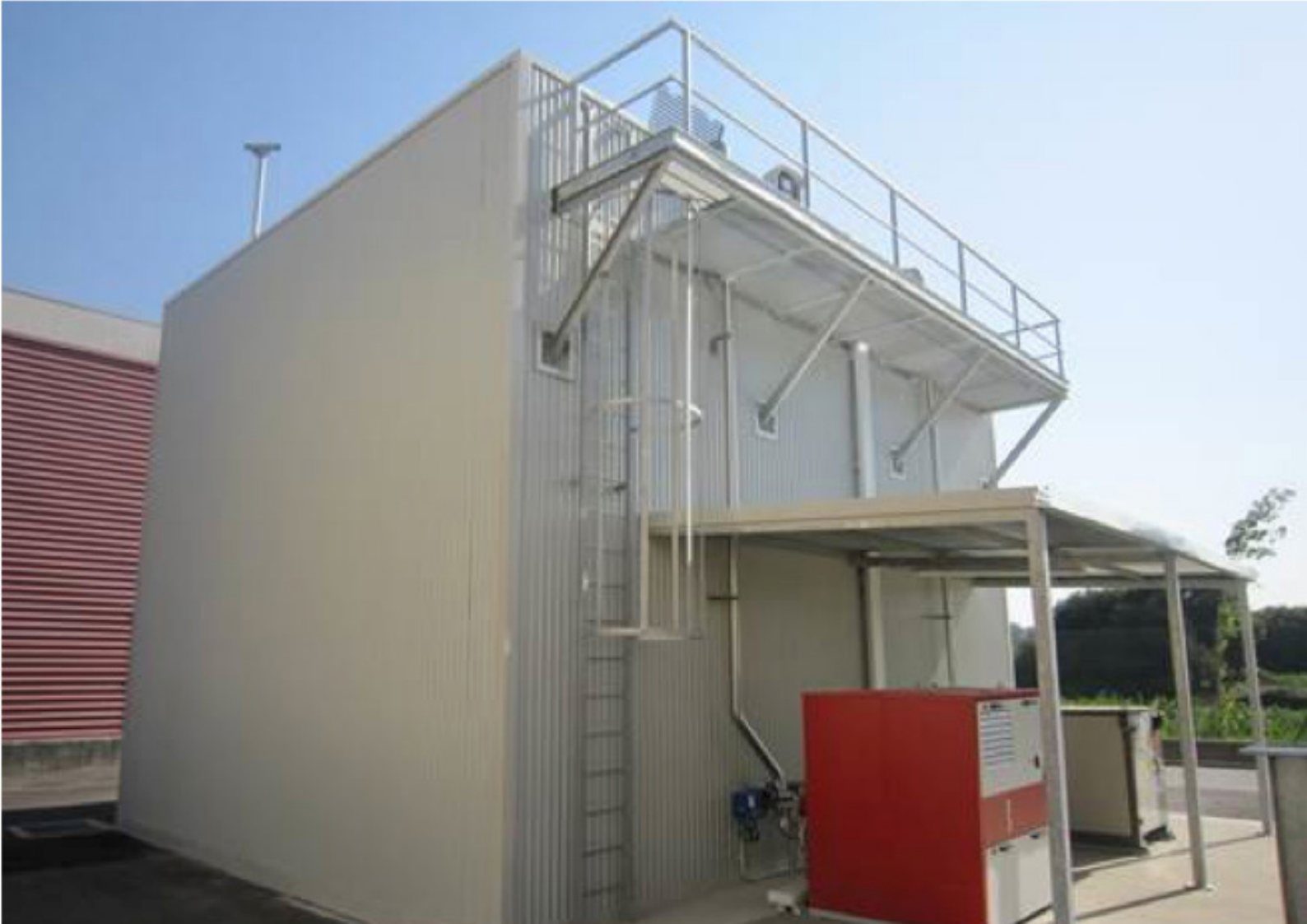
Outdoor view of the building housing the underground homogenising tank and the two ELAN® reactors which are part of the project.
